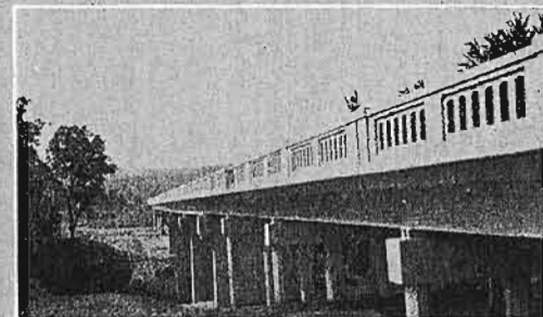
FOURCHE LA FAVE BRIDGE - ROUTES 9 AND 10, NEAR PERRYVILLE. 629' STRUCTURE REPLACING OLD INADEQUATE STEEL STRUCTURE.
